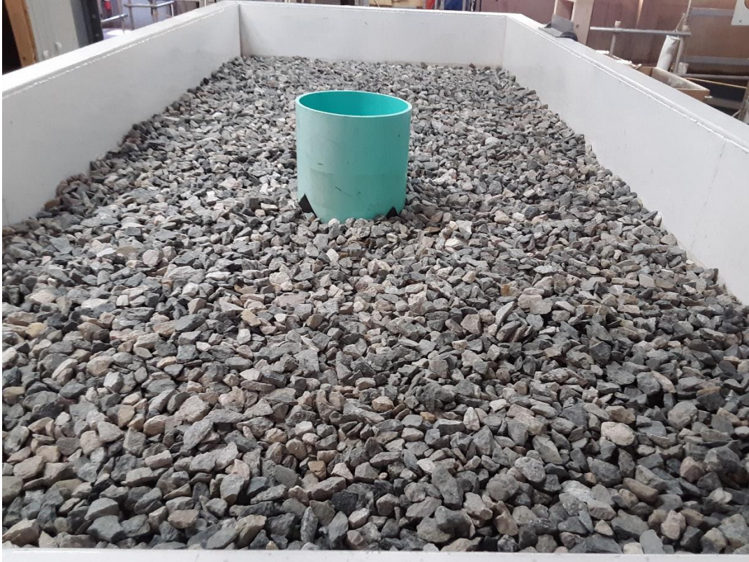
Figure 6 Installed R-Tank Treatment Row System
