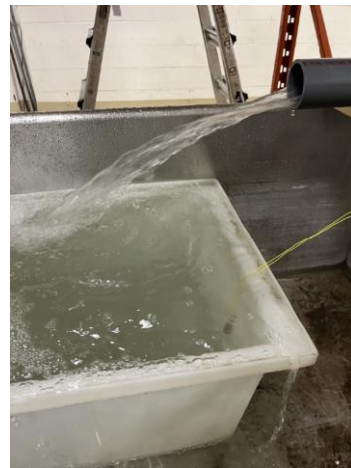
Figure 6 Effluent and Drawdown Sampling Point
