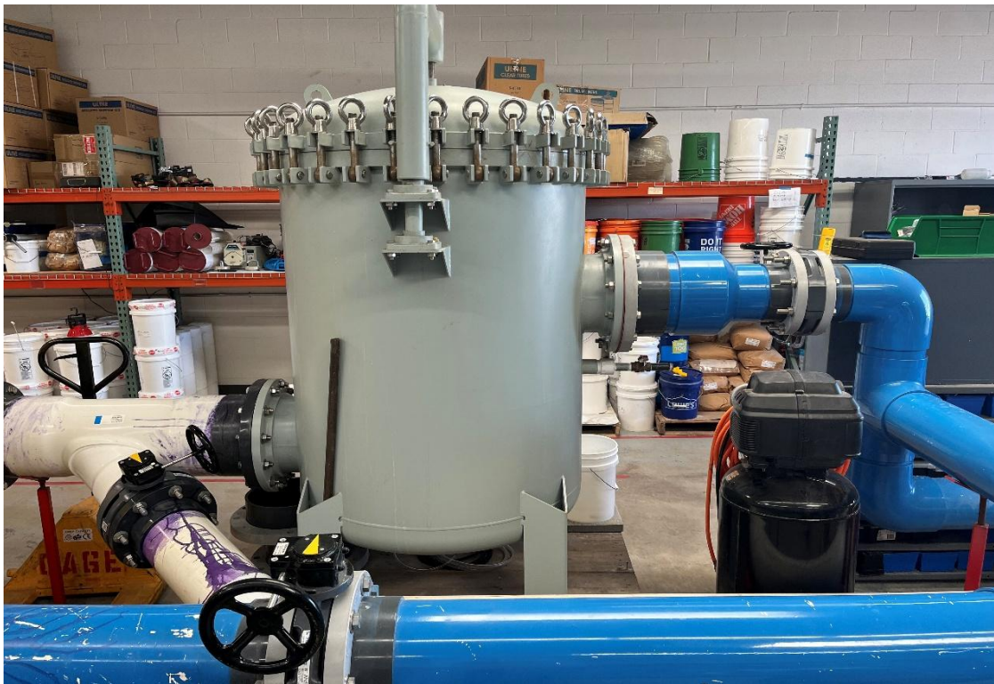
Figure 7: Test Loop Filter Vessel
