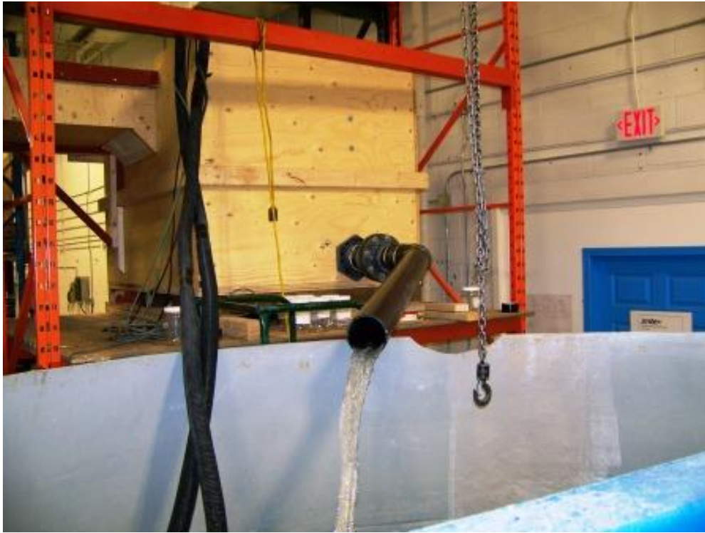
Figure 5 BioPod™ Biofilter Effluent Pipe
